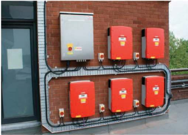
Figure 4: Commercial inverter bank (image courtesy of Planet Solar (NI) Ltd)
