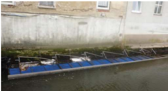
Figure 8; WSHP; closed loop river collector (Image courtesy of Dimplex, Germany)
