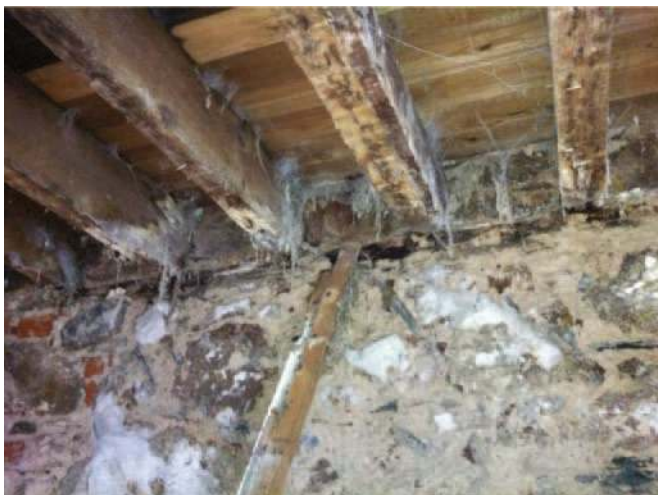
Figure 17: Rotten timbers at Inishcoo
