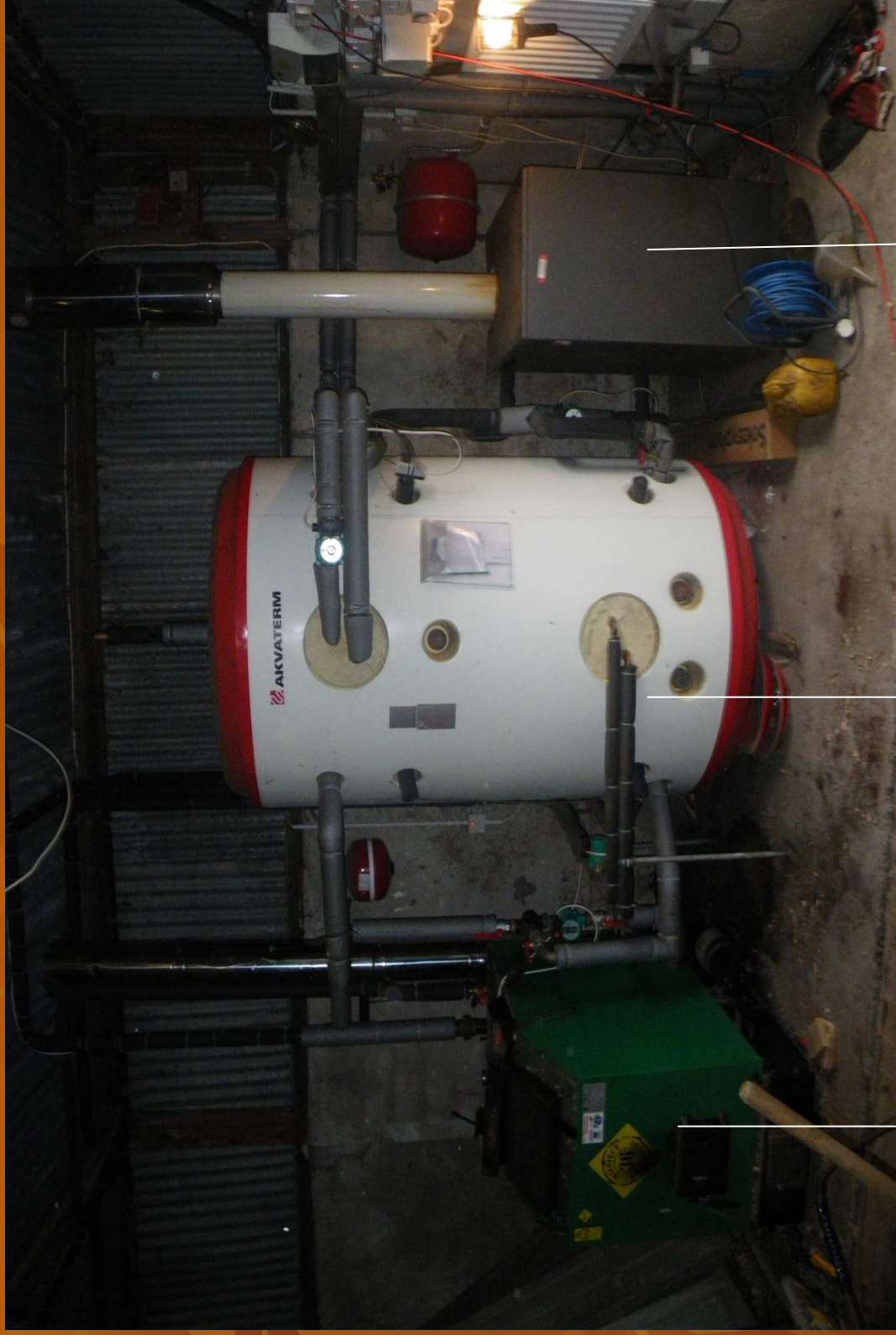
32kW Log Boiler
