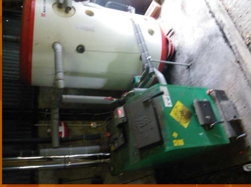
Log Boiler + Oil Boiler + Thermal Store
